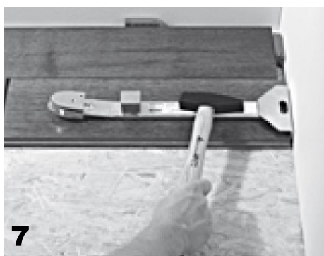
7. A pull bar or pulling iron can be used to help seat the end planks effectively
