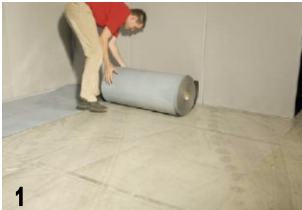
1 ROLL OUT THE EASYLAY OVER THE POLYTHENE MOISTURE BARRIER IN ROWS NEXT TO ONE ANOTHER (THE
