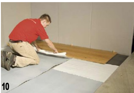
10 THE SECOND BOARD IS TAPPED INTO THE FIRST TO GIVE A TIGHT FIT, FOLLOWING THIS, THE SPARE FILM BETWEEN THE EASYLAY AND THE BOARDS IS REMOVED. FROM NOW ON WORK IS CARRIED OUT WITH THE ACTUAL PROTECTIVE LAYER OF EASYLAY
