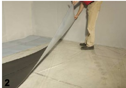
2 TURN OVER THE EASYLAY SO THAT THE SMOOTH PROTECTIVE LAYER IS ON THE UPPER SIDE
