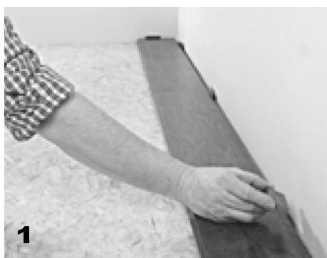
1. Cut the first row to size, centre and align the planking to the area
