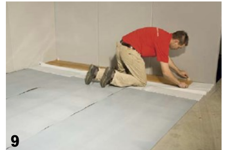
9 With wedges a minimum expansion of 10mm needs to be allowed, for larger rooms this needs to be increased.
