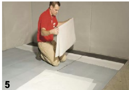
5 FOLD A PIECE OF FILM TAKEN FROM SOME SPARE UNDERLAY IN TWO, DON'T WORRY KEEP IT SAFE AND THE UNDERLAY CAN BE USED LATER
