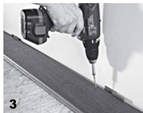
3. The planks in the first and last rows are fixed from the top with either nail or screw, the fixing is placed around 15mm from the edge of the plank
