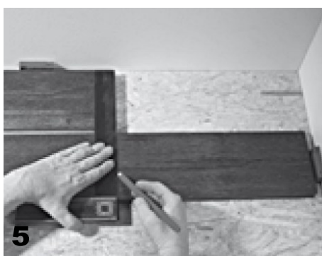
5. The row finishes by cutting your plank allowing for the expansion gap the cut off piece will return and start the second row
