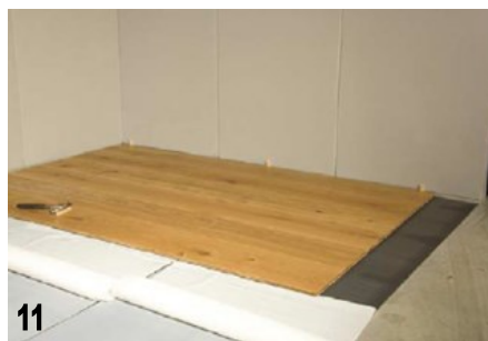
11 FROM HERE ONWARDS, SEVERAL ROWS CAN BE POSITIONED SEAMLESSLY BEFORE THE PROTECTIVE LAYER BETWEEN THE WOOD AND THE EASYLAY IS REMOVED
